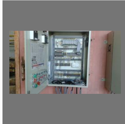
Electric PLC/RTU Panel
