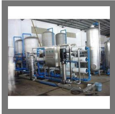
Sweet Water Treatment Plant Services
