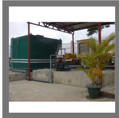
Industrial Water Treatment Plant Services
