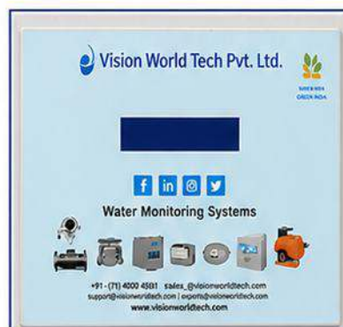
Control Interface Close-up
